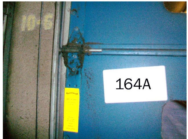
Figure 9.21: Lint accumulation on hardware
