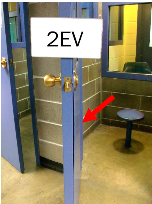
Figure 9.12: Door 2EV damaged door face
