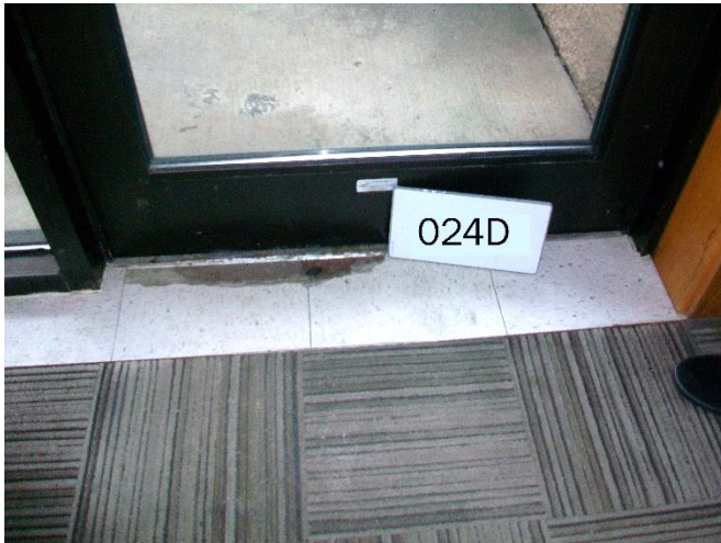
Figure 9.02: Door 024D showing damaged floor tiles.
