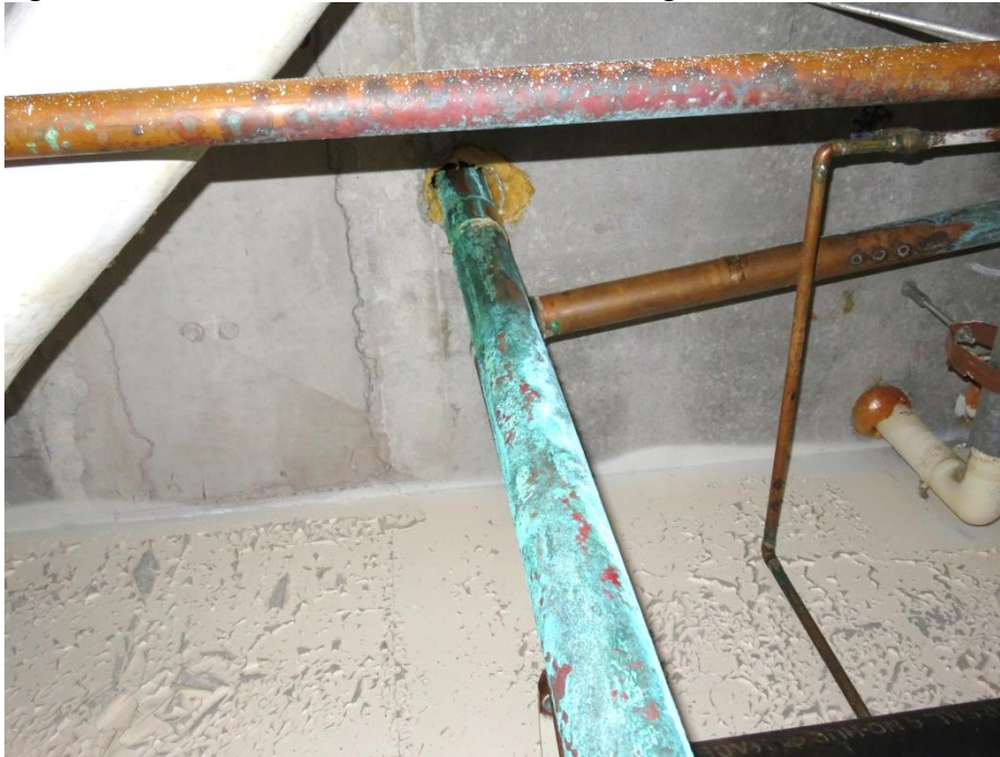
Figure 17.12: New clothes washer drain leak damage ( Basement Floor) inside the drain room
