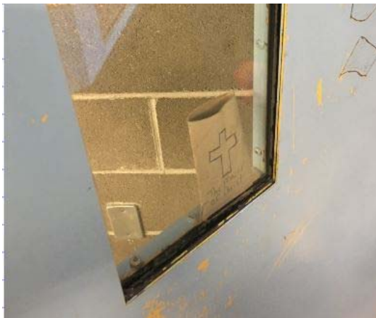
Figure 10.08: Glazing Stops Missing
