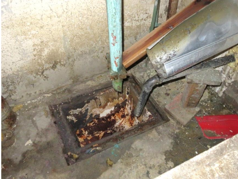
Figure 17.10: Clothes washer drain discharge (Basement Floor) inside drain room
