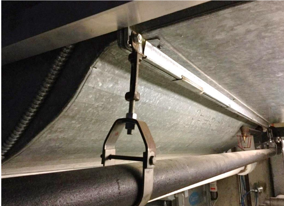
Figure 3/6.05: Example of suspended utility suspended from suspended utility.
