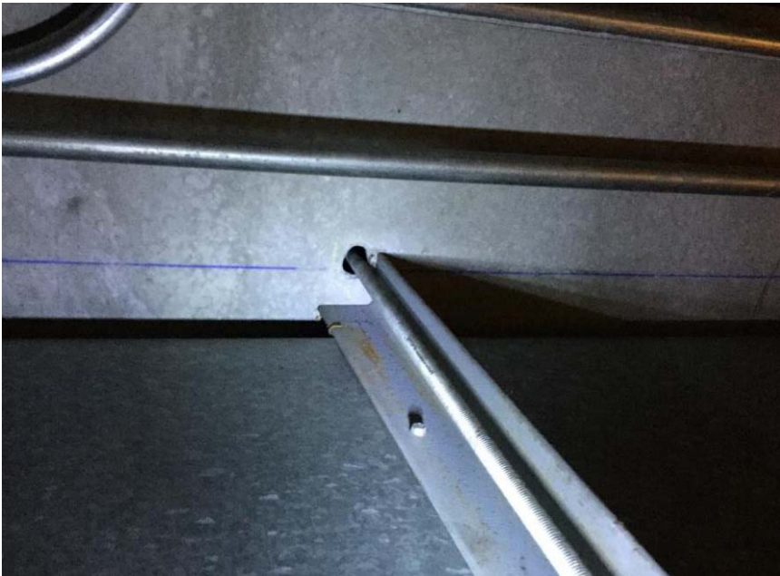
Figure 3/6.06: Oversized holes through the bottom of the overhead hollow core planks.
