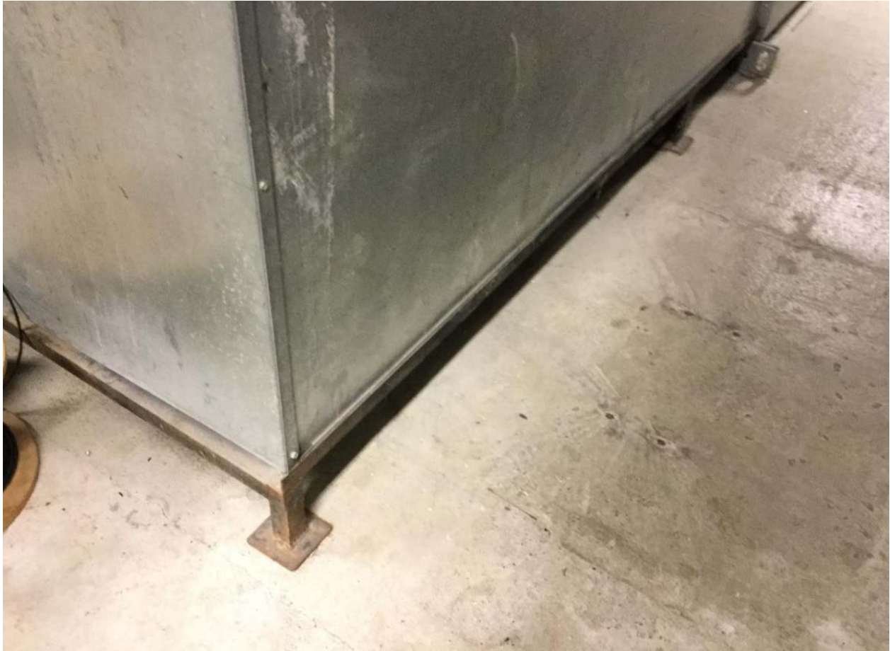
Figure 3/604: Unanchored equipment and duct supports.
