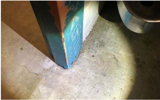
Figure 10.04: Rusted Frame at Base
