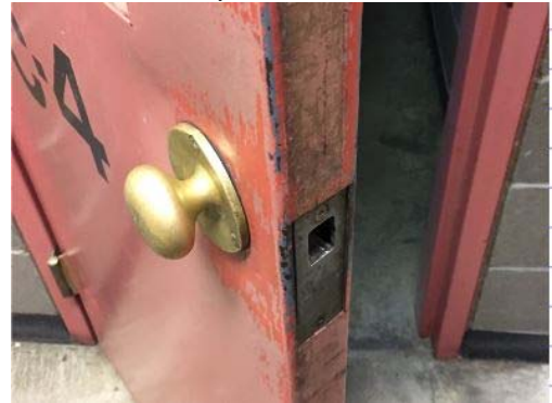
Figure 10.02: Denting at Door Knob/Door Bulging at strike plate
