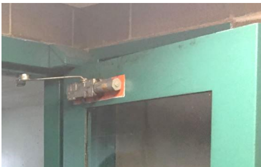
Figure 10.14: Door Closer Leaking Oil
