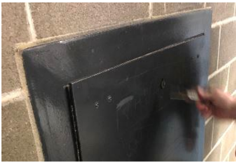
Figure 10.13: Bent Mechanical Chase Door
