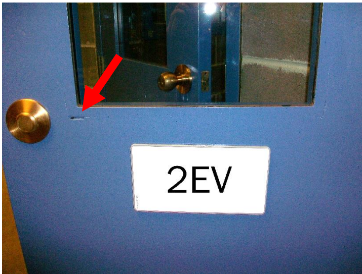
Figure 9.14: Door 2EV-Typical damage at vision lite frame
