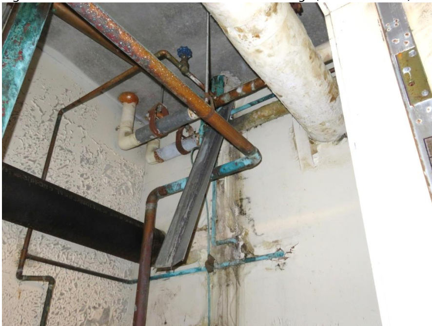
Figure 17.11: Older clothes washer drain leak damage (Basement Floor) inside the drain room
