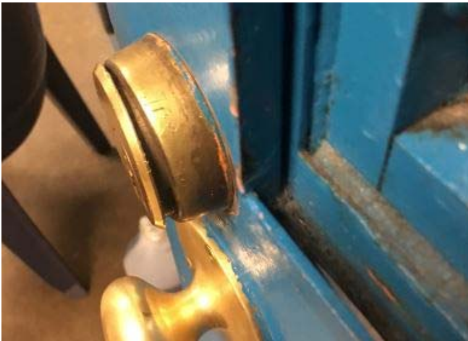
Figure 10.03: Damaged Mogul Lockset
