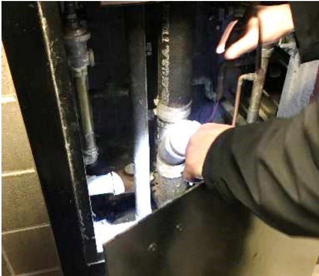
Figure 10.06: Dust Accumulation in Mechanical Shaft
