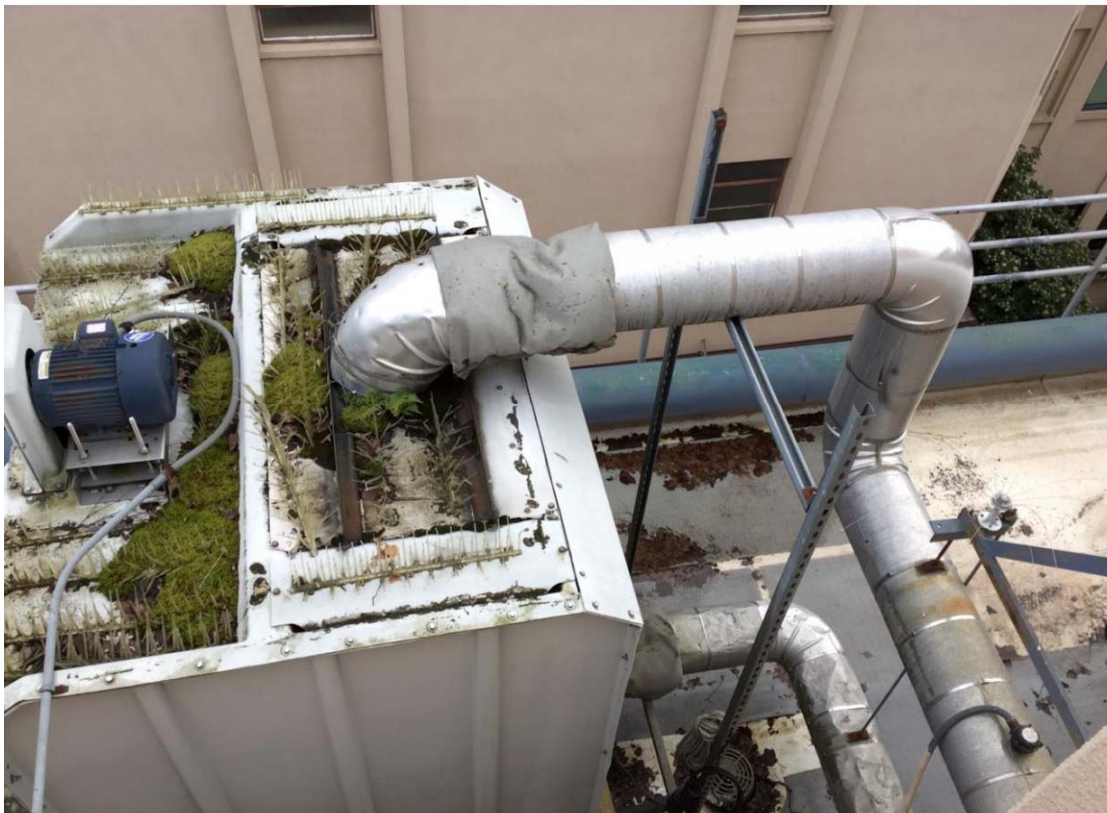
Figure 3/6.02: Cooling tower on cantilevered support close to the edge of the roof and 5" pipes that are not seismically restrained.
