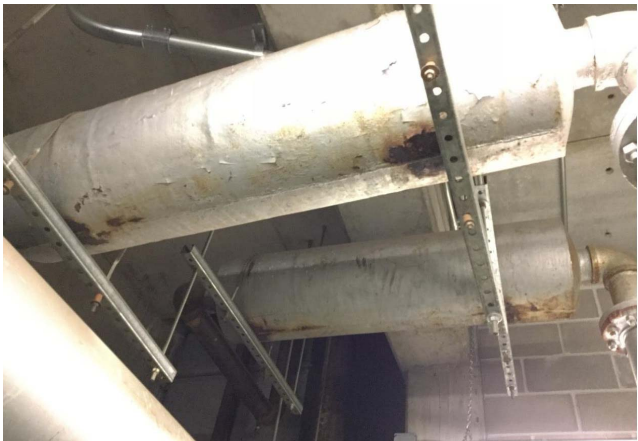
Figure 3/607: Unbraced mufflers and exhaust pipes for emergency generators.
