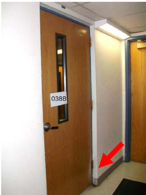
Figure 9.06: Door 038B shows signs of damage at wall and loose base.
