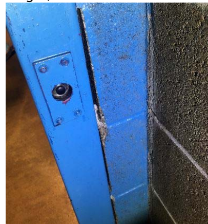
Figure 10.17: Missing Groove Bulging at Strikeplate
