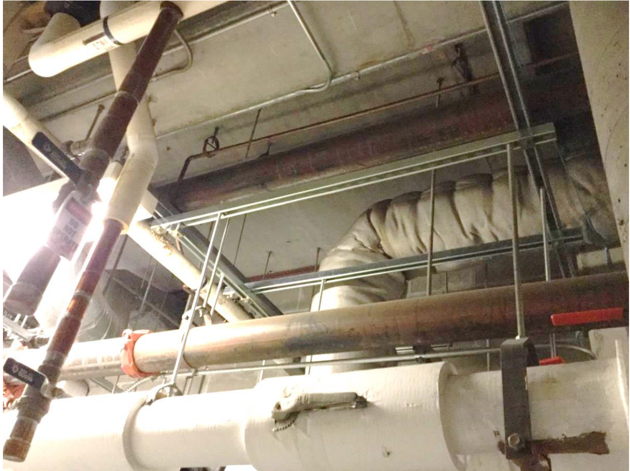
Figure 3/609: Unbraced pipes and ducts. Suspended utilities hanging from suspended utilities.
