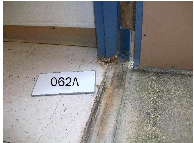
Figure 9.05: Door 062A showing condition of threshold and frame
