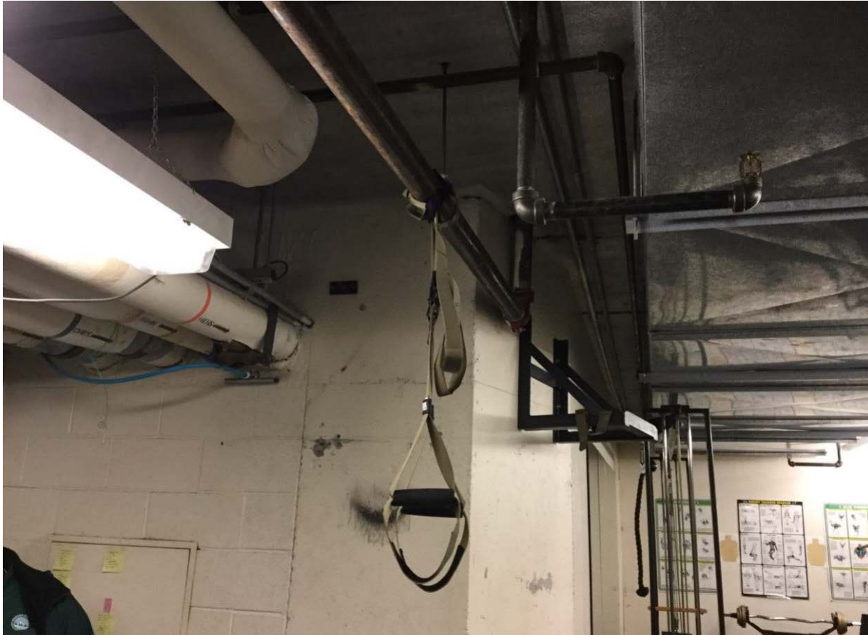
Figure 3/6.10: Suspended utilities used for hanging supports.
