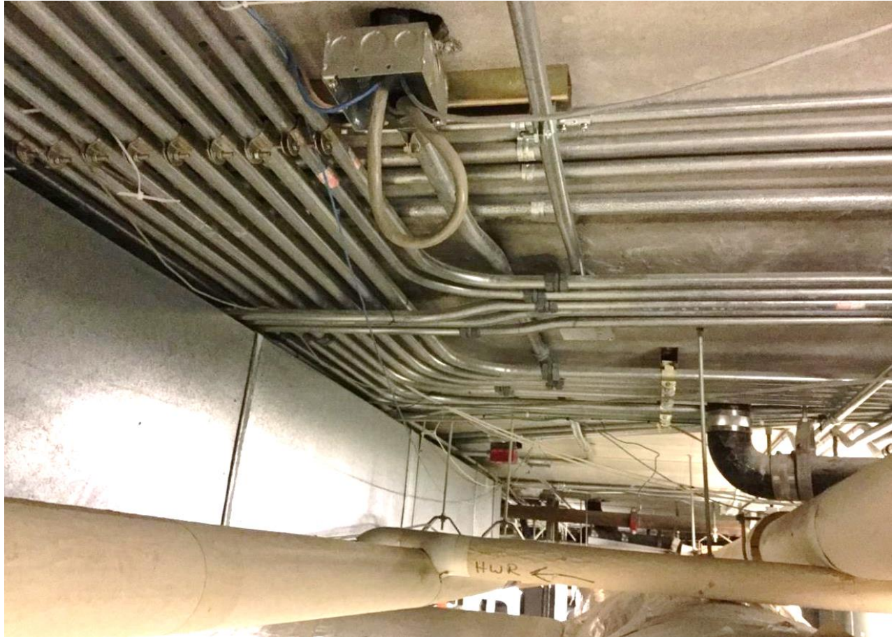
Figure 3/6.03: Unbraced pipes and ducts. Overhead obstructions will interfere with anchorages.
