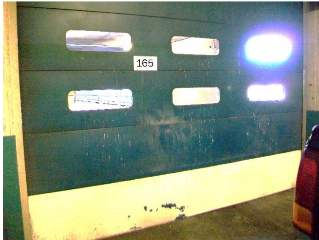
Figure 9.20: Damage at bottom door panels
