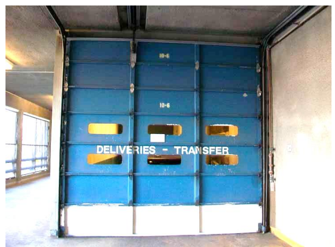
Figure 9.18: Condition of overhead panel door
