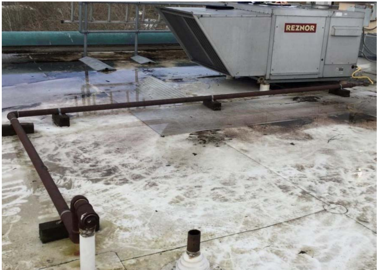
Figure 3/6.01: Unsecured rusty gas pipe on roof.
