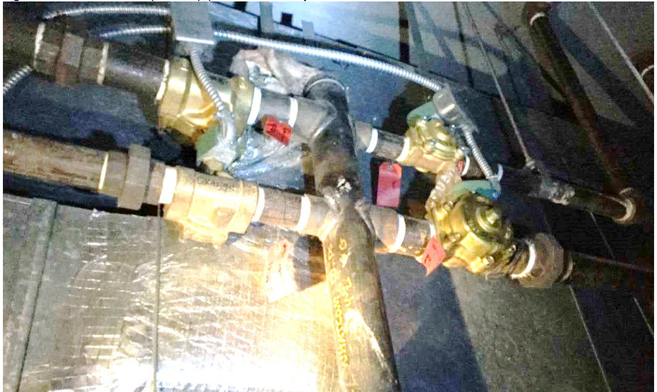
Figure 3/6.13: Unbraced sprinkler pipe valve assembly.
